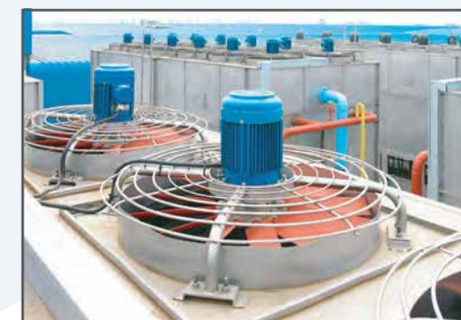
Fan and water pump
